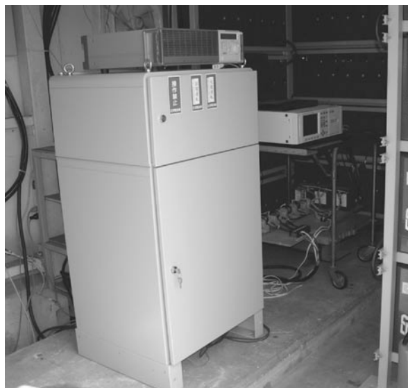
図7 蓄電システム (針貝工場) Fig.7 Electric power storage system (in HARIGAI Factory)
