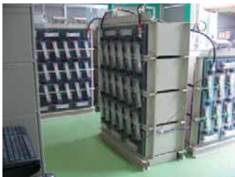
図9 蓄電システム Fig.9 Electric Power Storage System
