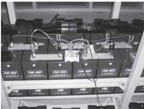
図9 鉛電池列外観 Fig.9 Appearance of VRLA batteries string
